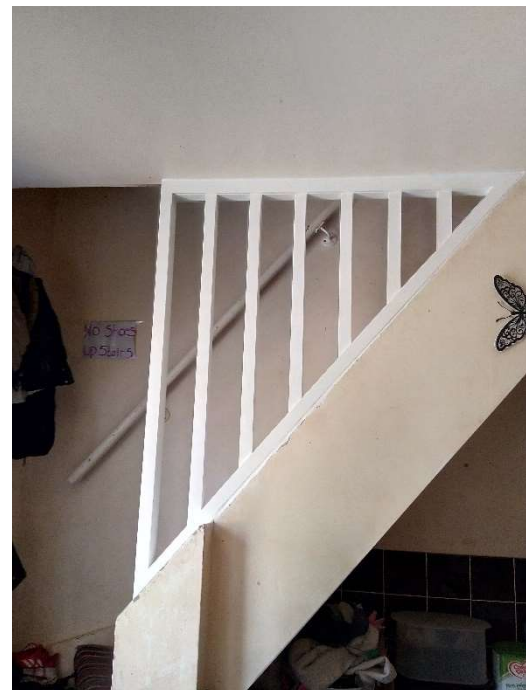
(photo after guardrail compliance after Building Act Notice was served)
